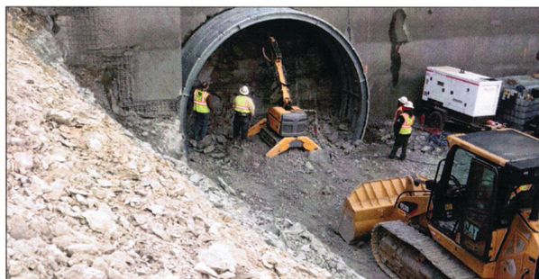
A Brokk robotic excavator fitted with an Atlas Copco hoe ram was a primary piece of equipment in the construction of the tunnel.
